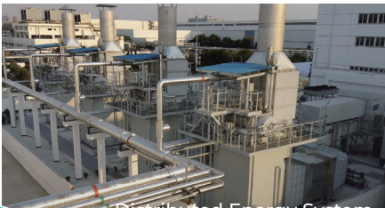
Distributed Energy System
